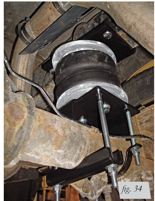
Right side (passenger): rear view of installation.
