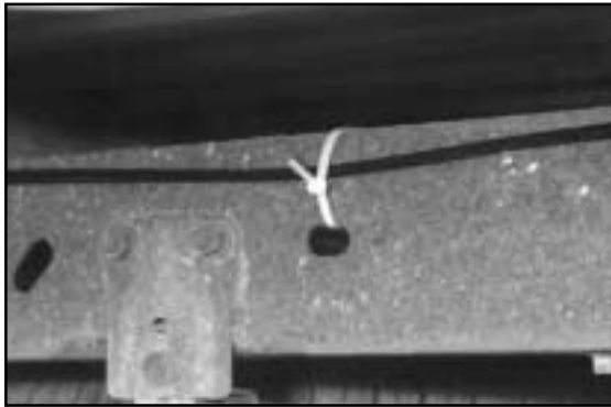
Inspect air lines to be sure it is not pinched. Tie straps may be too tight. Loosen or replace strap. Replace leaking components.
