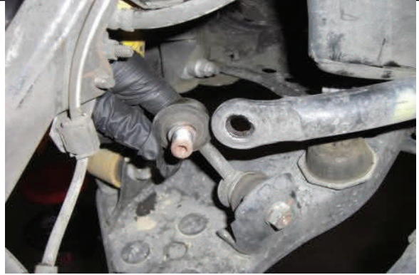
Disconnect both sides sway bar end links
